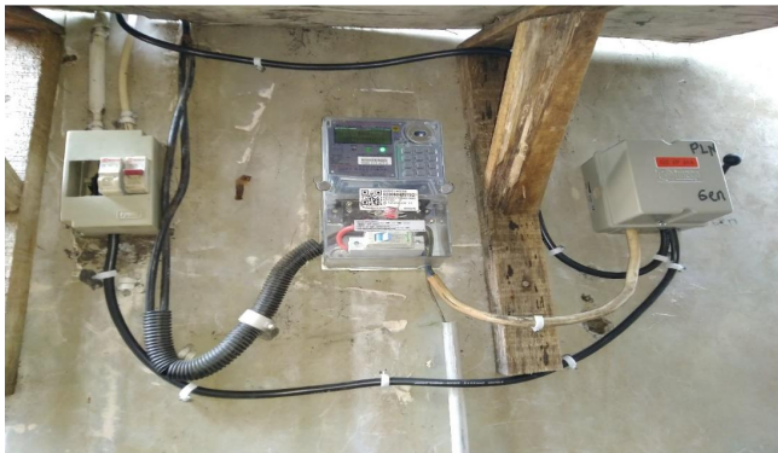
Gb. 1. KWH meter serta handel PLN/Genset
