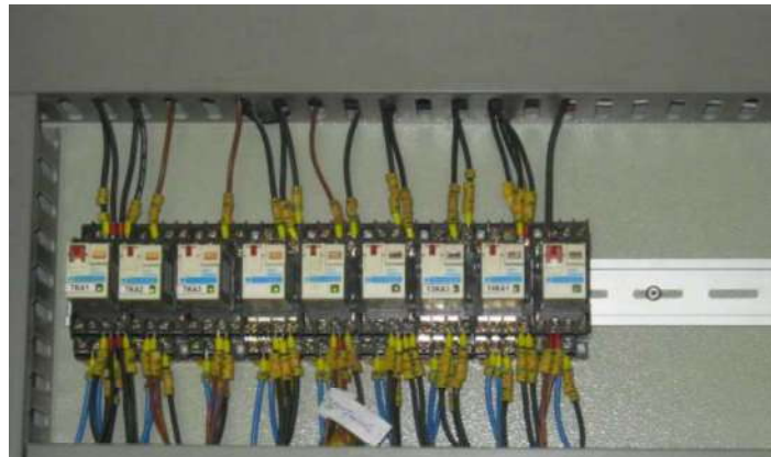
Gambar 3.11 Interface PLC zelio
