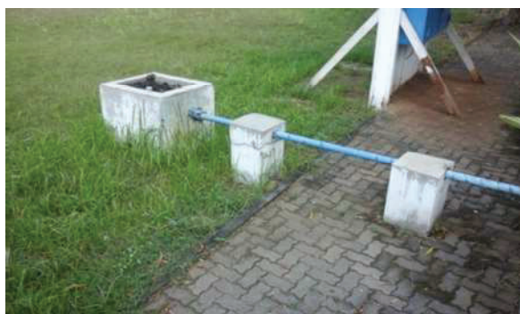
Fig. 6. Location of submersible pump.
