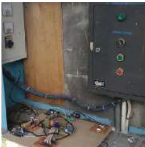
Fig. 7. Control system for submersible pumps.
