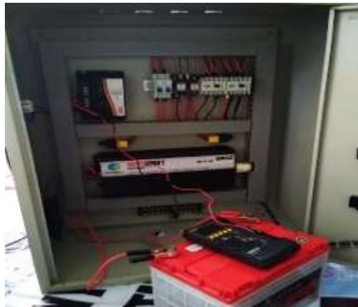
Figure 6. Device system off grid
